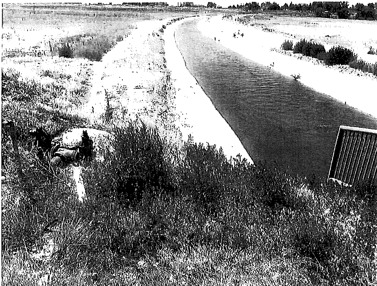
Section of water line to be modified to discharge into the Ridenbaugh Canal.
